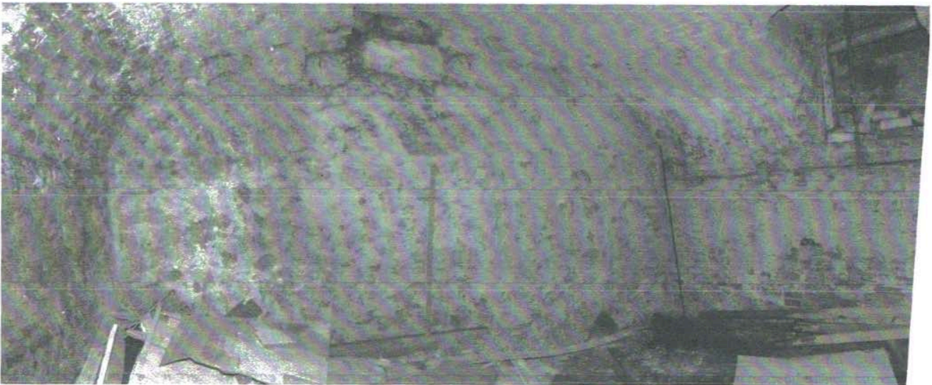
View of the end wall of the cellar of the pizza take away.
